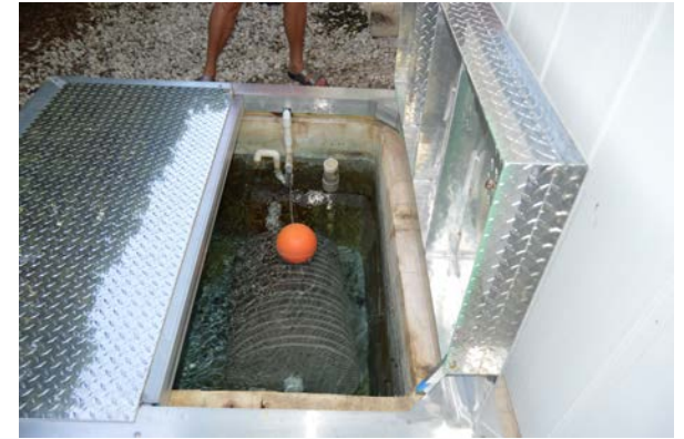
POOL FILTER EQUIPMENT / ENCLOSURE
