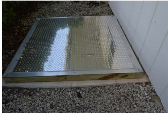
POOL FILTER EQUIPMENT / ENCLOSURE
