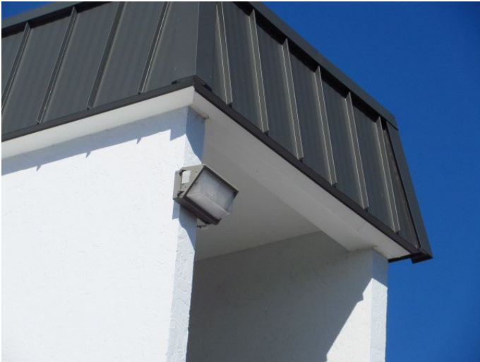
VIEW OF EXTERIOR LIGHTING
