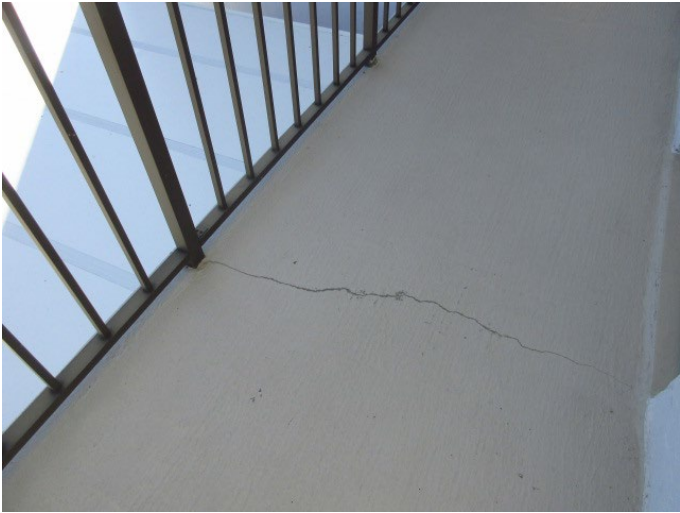
VIEW OF CRACK AT ELEVATED WALKWAY
