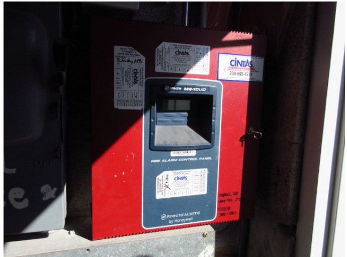
VIEW OF CENTRAL ALARM PANEL
