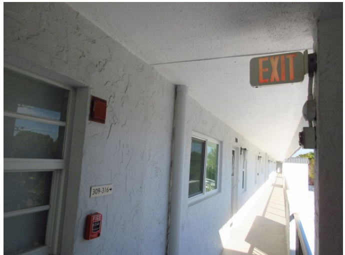
VIEW OF LIFE SAFETY EQUIPMENT
