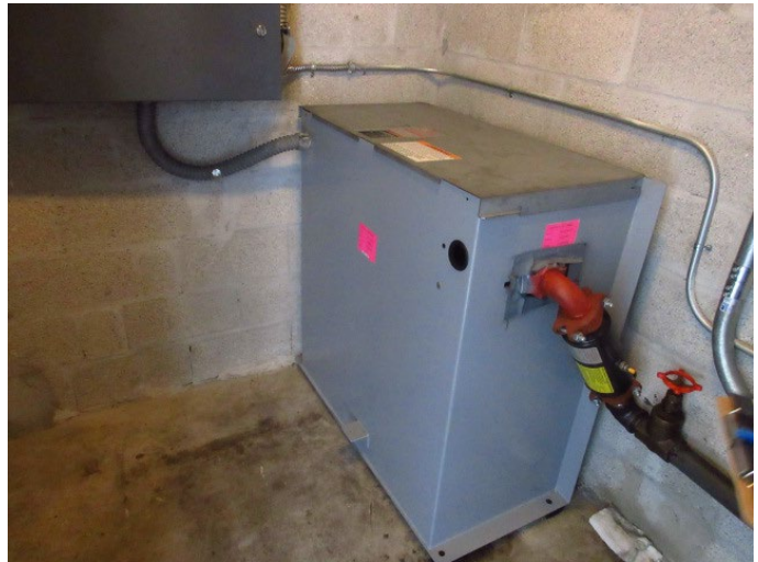
VIEW OF ELEVATOR EQUIPMENT
