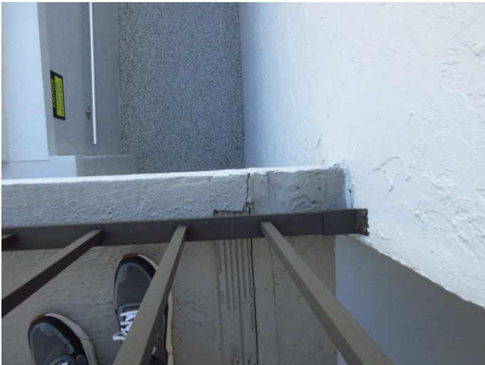
VIEW OF FAILING EXPANSION JOINT
