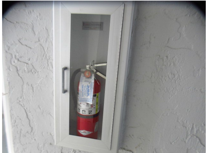
VIEW OF FIRE EXTINGUISHER
