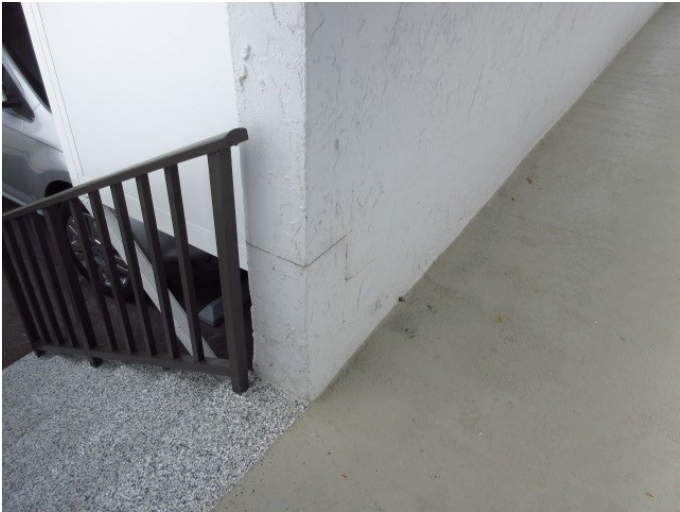
VIEW OF CMU STEP-CRACKING
