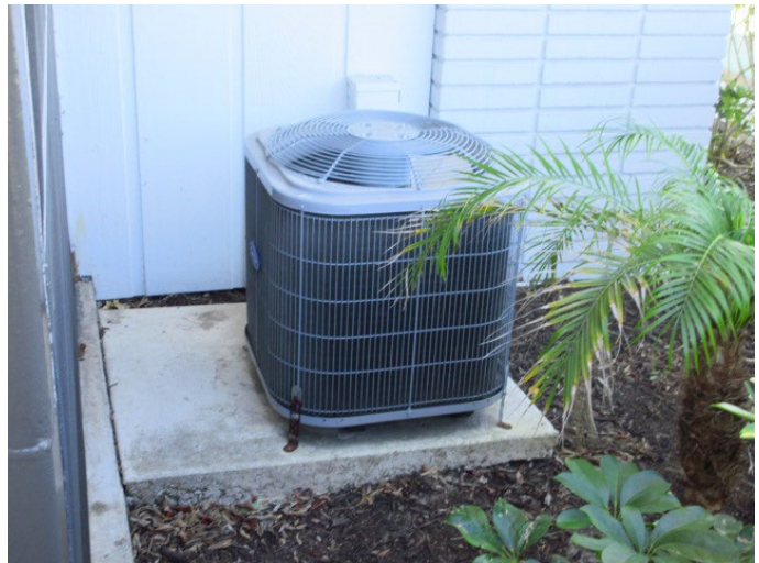
GENERAL VIEW OF HVAC EQUIPMENT
